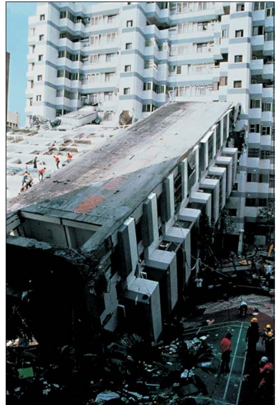
The building has tilted as a result of column failure & has partly damaged the nearby building (Taiwan 1999). (By Bachmann H., Sesimic Conceptual Design of Buildings)
